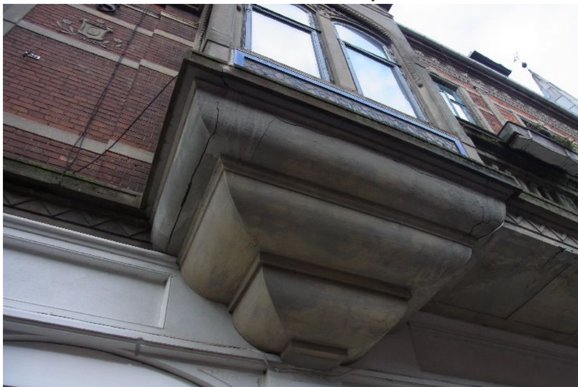
Revner i underside karnap
